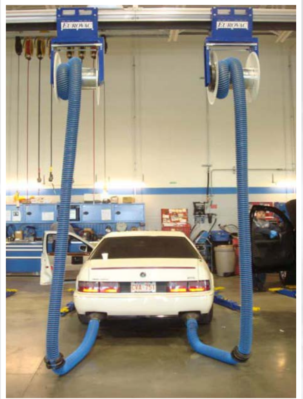
Spring hose reels and trolleys on rail
