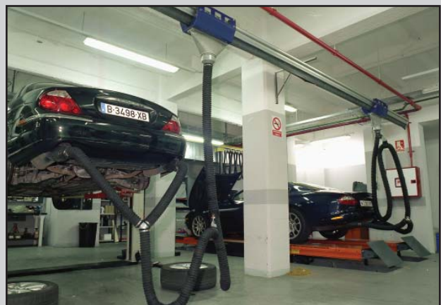
The Eurovac system can also be used with hose drops. A complete line of exhaust accessories are available.
